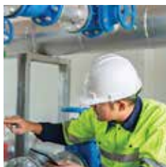
Hard Facilities Management
